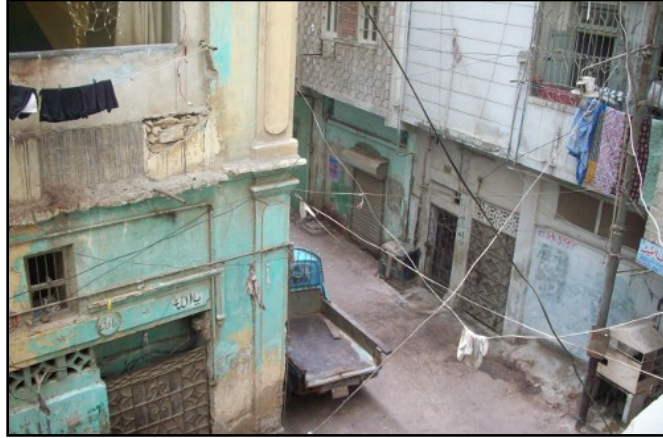
Fig. 19: Urban fabric of Lyari - narrow streets and alleys framed by decaying, dilapidated buildings. Source: Google Images.
