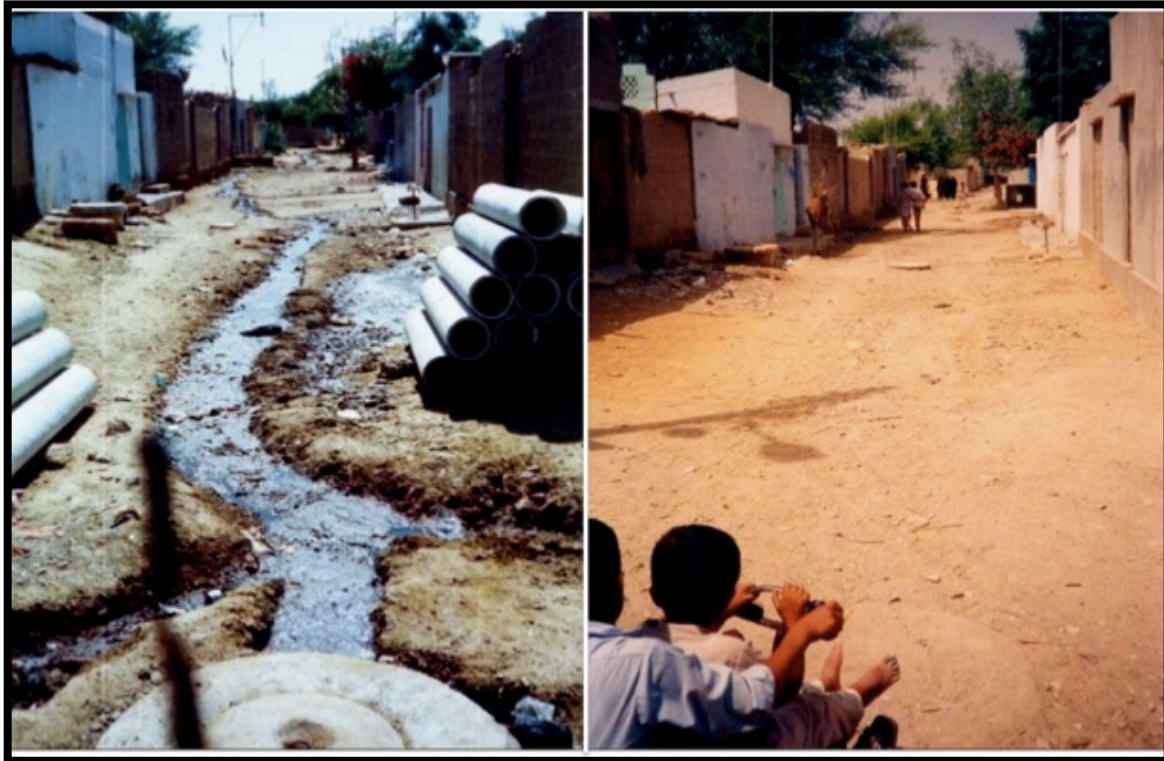
A lane in Orangi before and after the construction of sewer lines. Courtesy of OPP-RTI.
